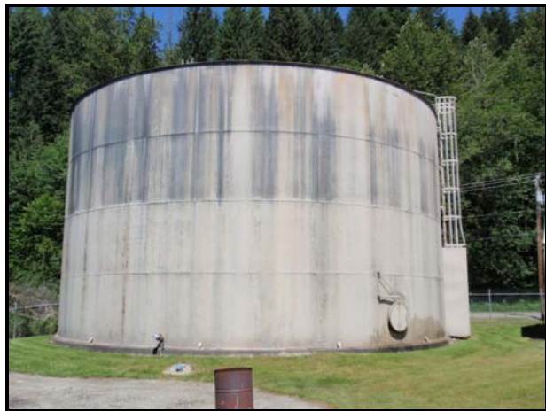
Water Treatment Plant Backwash Supply Storage Tank
