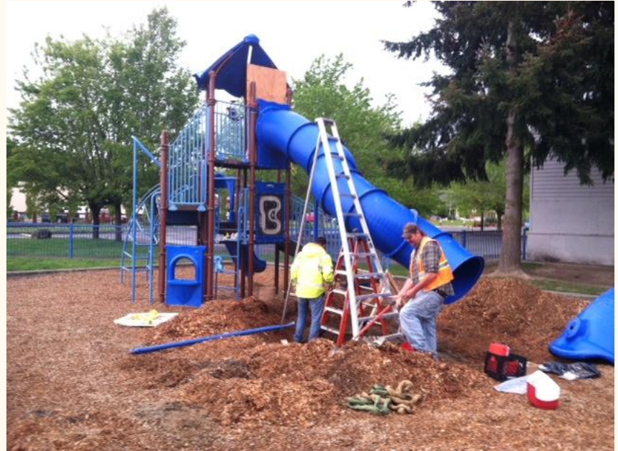
City staff Scott Cox and Brett Enders installing the new slide at the Boys and Girls Club
