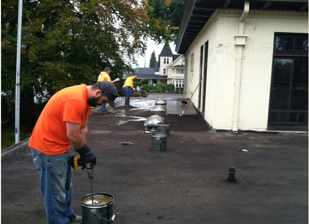
Chris Soren applying a coating on the roof in an effort to plug all the leaks in the old roof.
